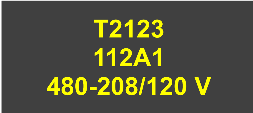
Figure 20. Transformer plate/label; 7/8-inch-high yellow letters on 4-inch high by 9-inch-wide black background (figure is approximately 1/2 scale). I&O is responsible for labeling high-voltage transformers (TH).
