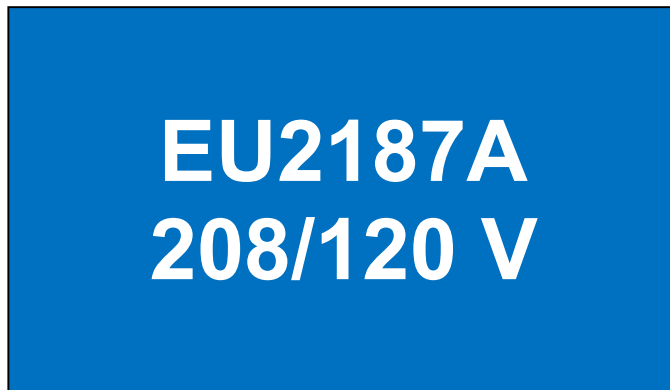
Figure 19. Distribution panel providing emergency uninterruptable power source (UPS) entry plate/label; 7/8-inch-high white letters on 4-inch-high by 7-inch-wide blue background (figure is approximately 1/2 scale)
